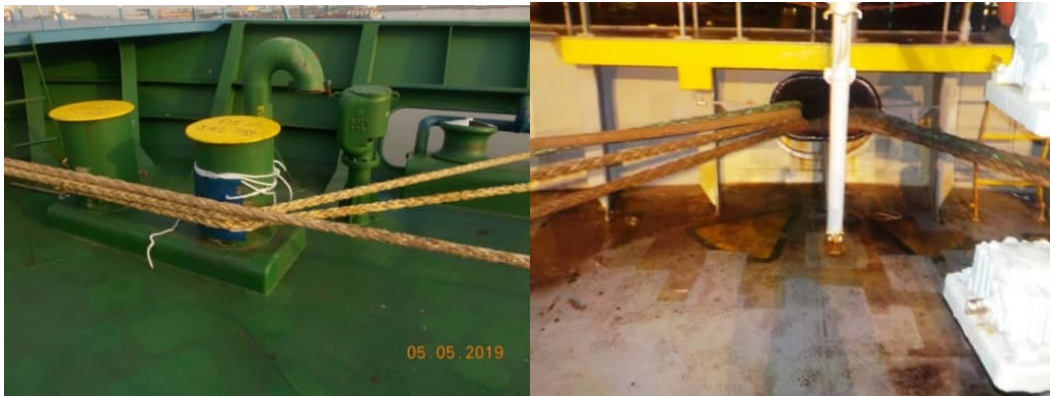
Fig 13: Overloading Fairleads and mooring bitts
