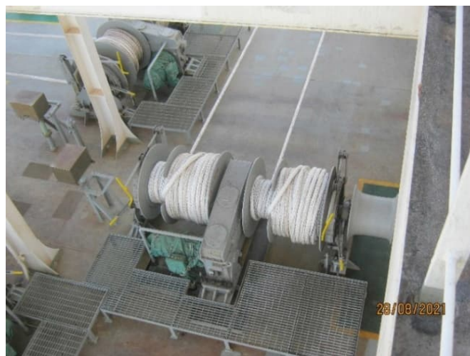
Fig 14: Multiple layers on a split mooring drum
